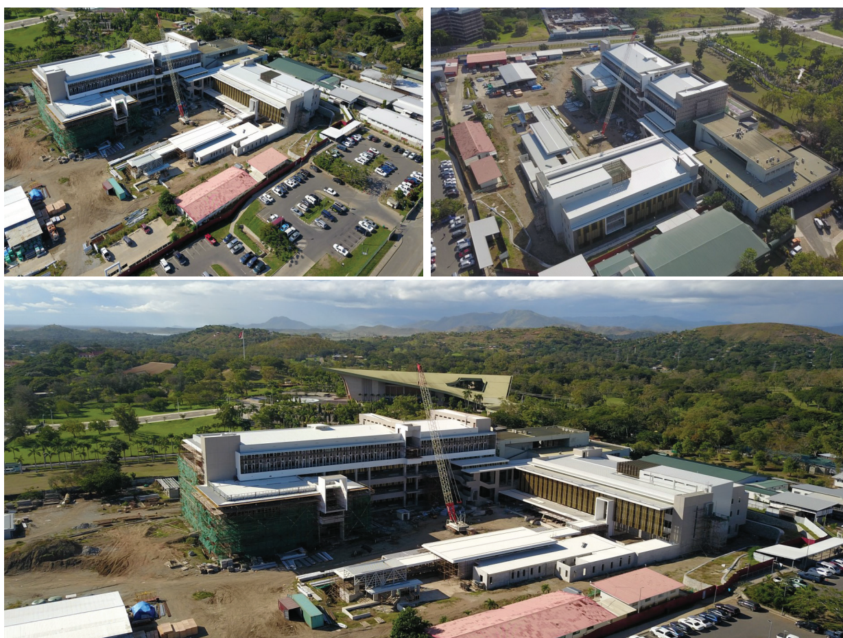
Aerial Images of the Waigani Supreme and National Court Complex work under progress. It is expected to be completed by year 2022.
